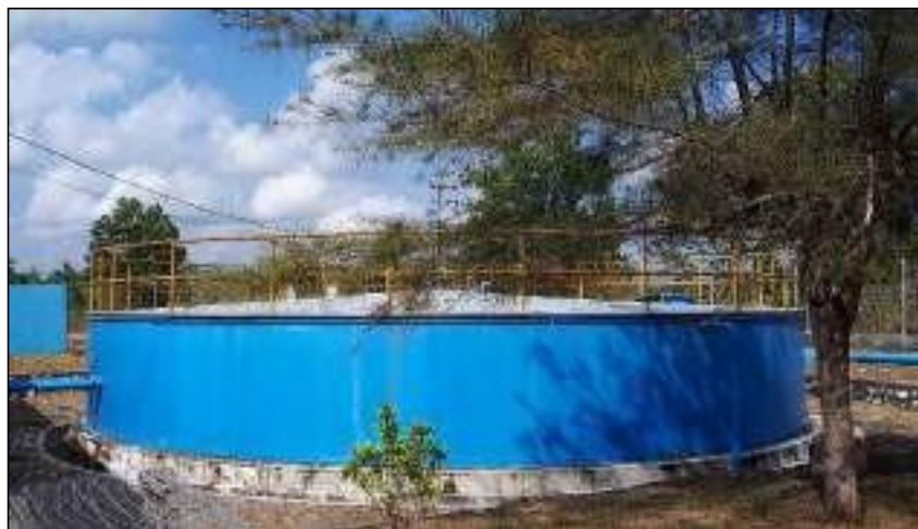
Gambar 3.47 Reservoir Perawas I Kapasitas 150 m 3
