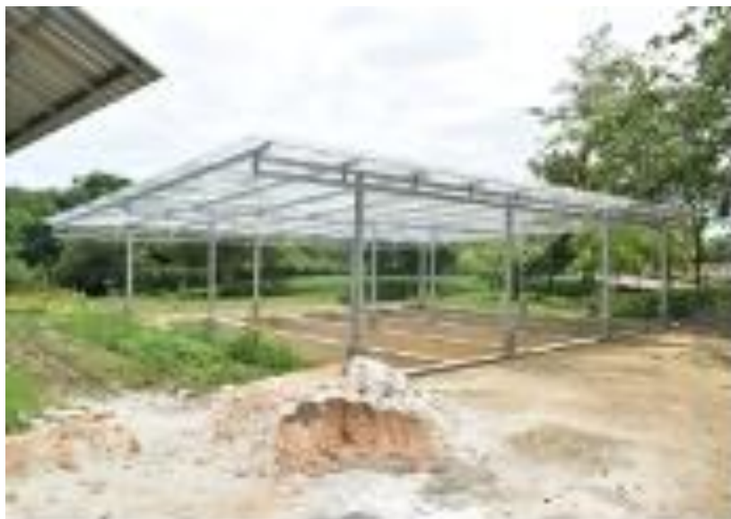
Sludge Drying Bed
