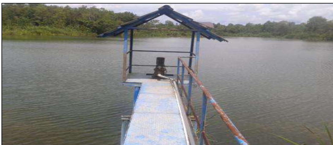
Sumber: Penyusunan Masterplan Distribusi Pelayanan PDAM, 2016 Gambar 3-84 Intake SPAM IKK Badau
